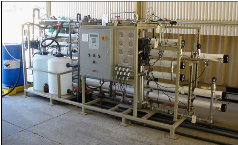
Figure 2-6. RO Pilot Unit
