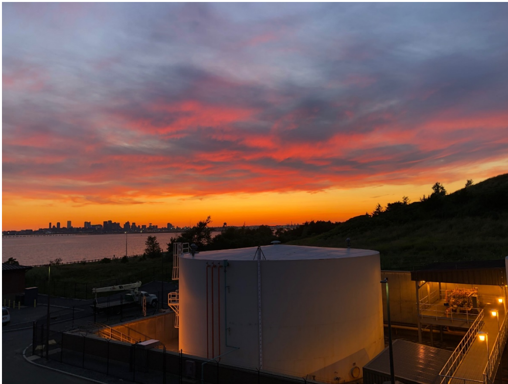
Deer Island Treatment Plant Thermal Power Plant
