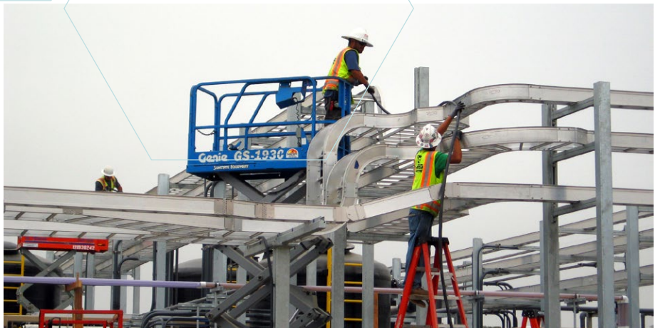
Cable trays being installed at the Regional Recycled Water Advanced Purification Center – a demonstration plant expected to be complete in early 2019.
