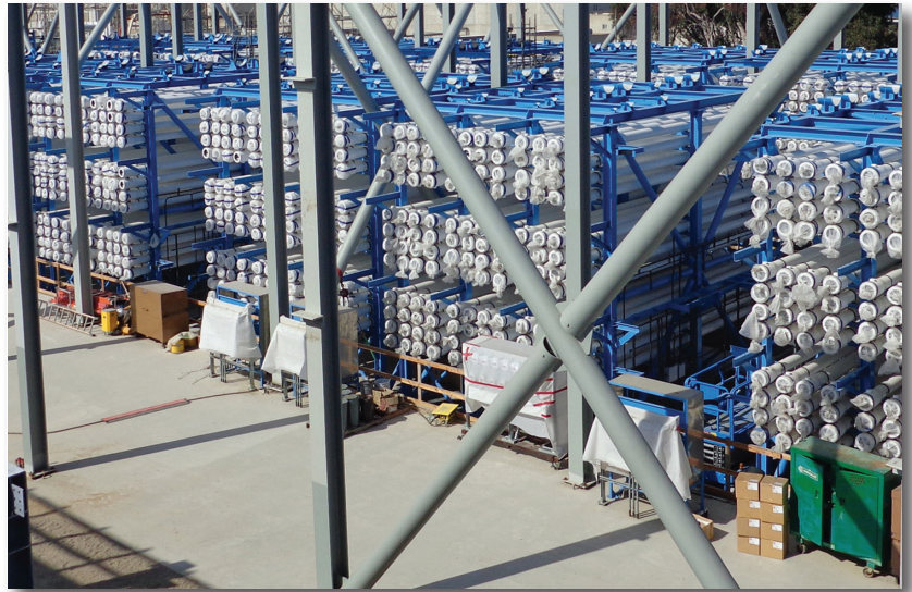
Reverse osmosis vessels are a key part of the desalination process.
