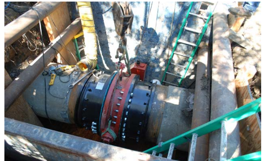
Newly installed valve
