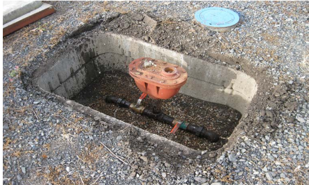
Old Style 2" Air Valve in Below Ground Vault
