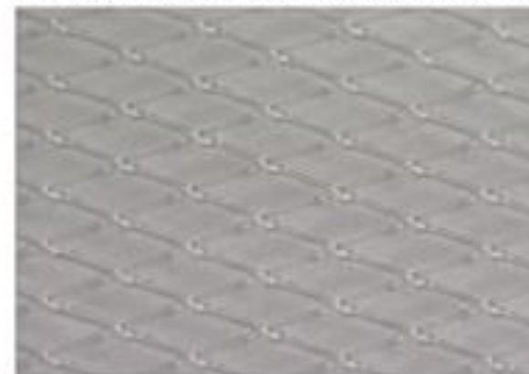
FEED SPACER CLEAN AND INTACT
